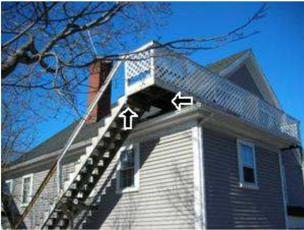
2.4 Picture 3 Lack of support for both decks in this area
