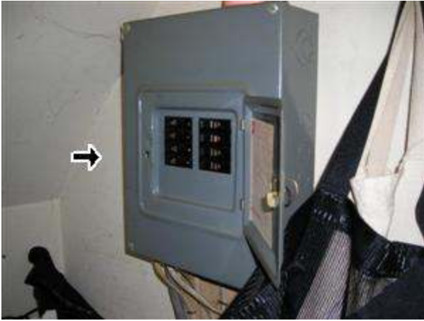
5.31.C Picture 1 Main electrical panel
