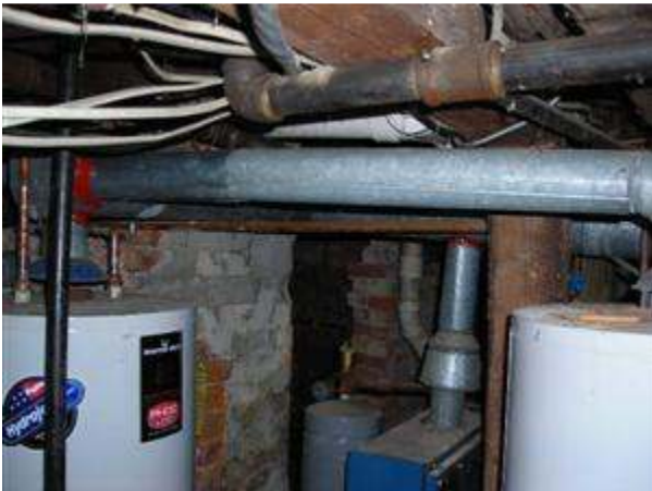
5.17.C Picture 3 Heat and hot water units for 19A & 19B
