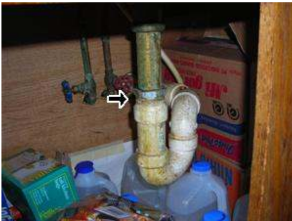
5.7.D Picture 1 Drain for the kitchen sink leaking
