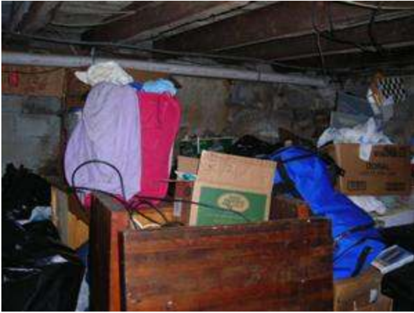
3.3 Picture 3 Limited visibility due to stored items
