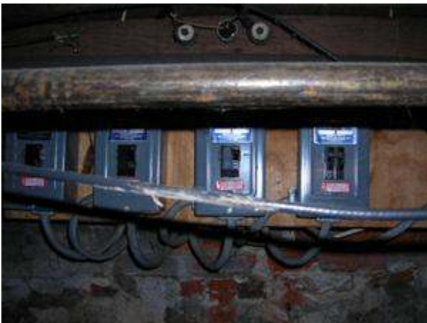
6.6 Picture 1 Main disconnect for each unit is in the basement
