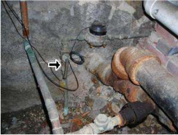
4.3 Picture 1 Water main shut off vlave
