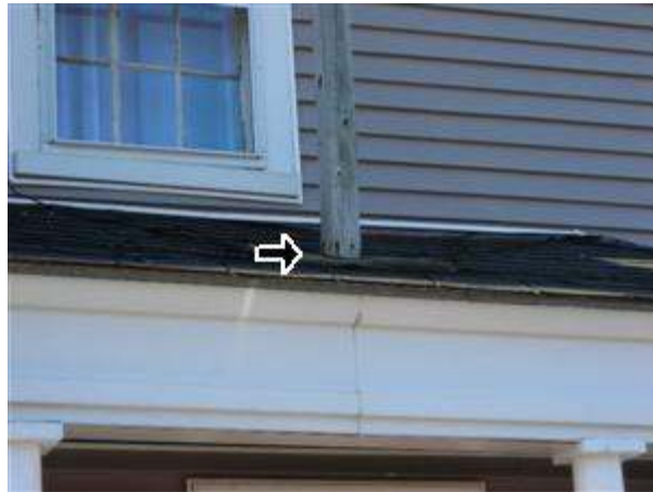
2.4 Picture 2 Deck not supported properly
