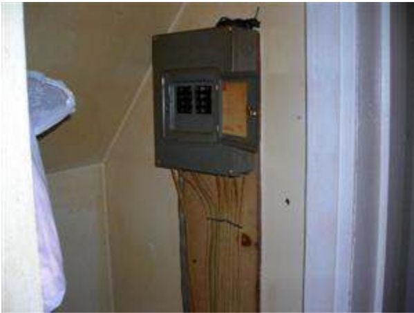
5.31.A Picture 1 Main panel located in closet
