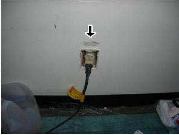
5.9.C Picture 3 Missing outlet cover
