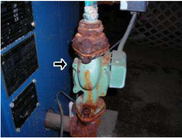
5.17.A Picture 1 Past evidence of water leaking at the circulating pump.
