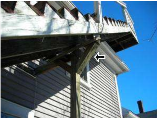
2.4 Picture 5 improper support for stairs
