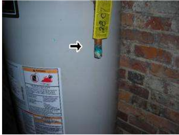
5.17.B Picture 2 Pressure relief valve should extend to the floor
