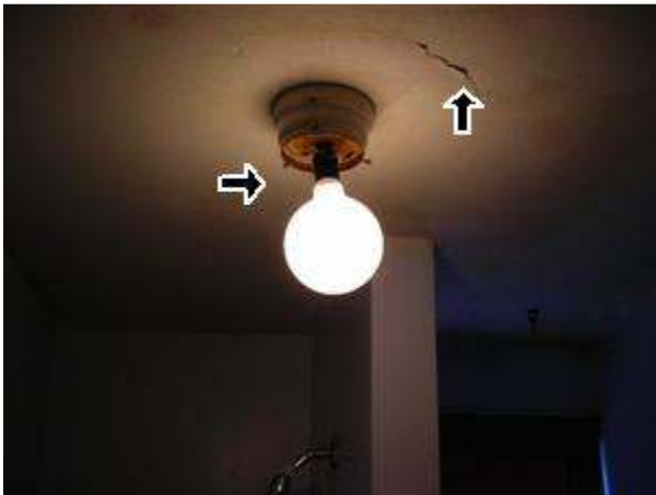
5.9.C Picture 1 Globe missing from light fixture/ ceiling repair, typical throughout the building
