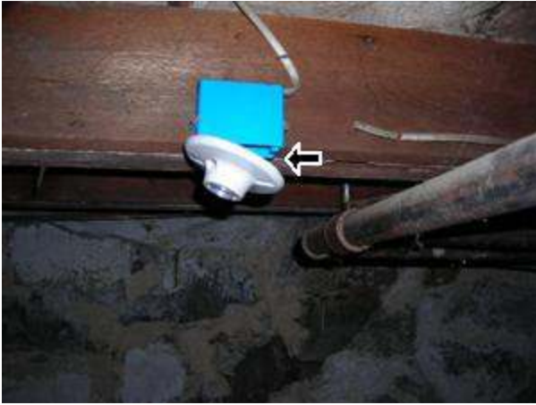
6.3 Picture 1 Light fixture in basement needs repair by a licensed electrician.
