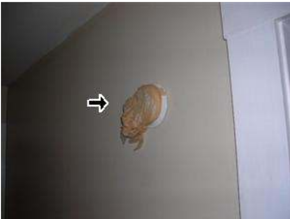
5.32.A Picture 1 Smoke detector/bag covering it.
