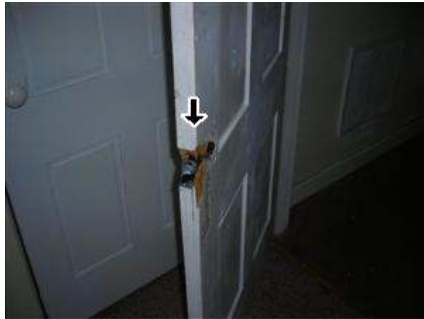
5.3.B Picture 2 Broken door/missing passage set
