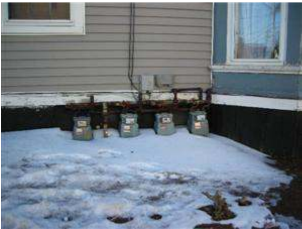
4.4 Picture 1 Gas meters on exterior, this area should be clear and accessible
