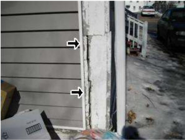
2.4 Picture 9 Rear corner board needs repair
