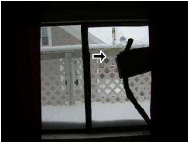
5.4.B Picture 1 Broken window
