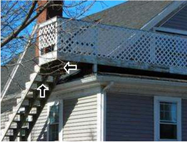
2.4 Picture 7 Lack of support
