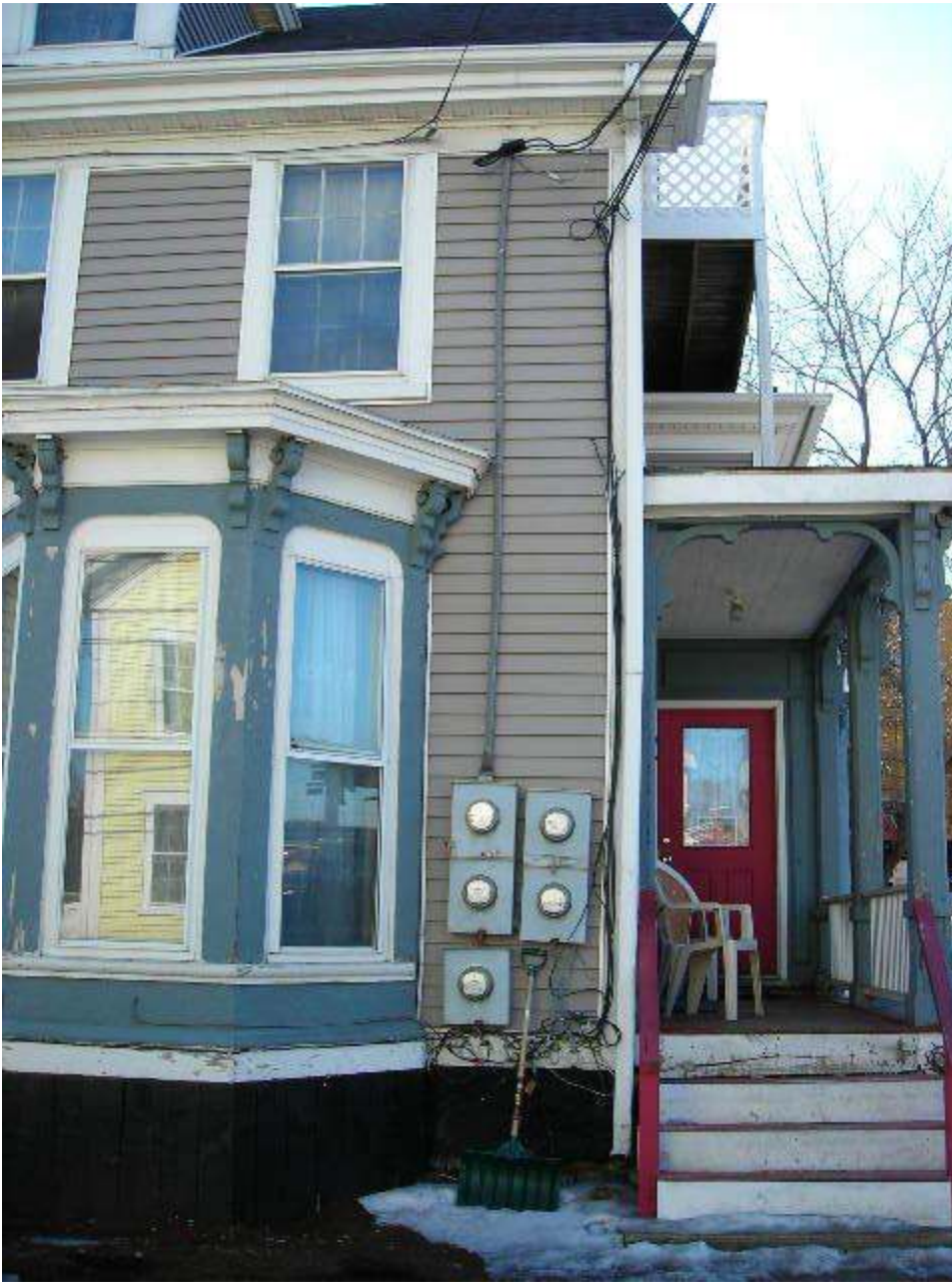
6.0 Picture 1 200 amp service entry into building
