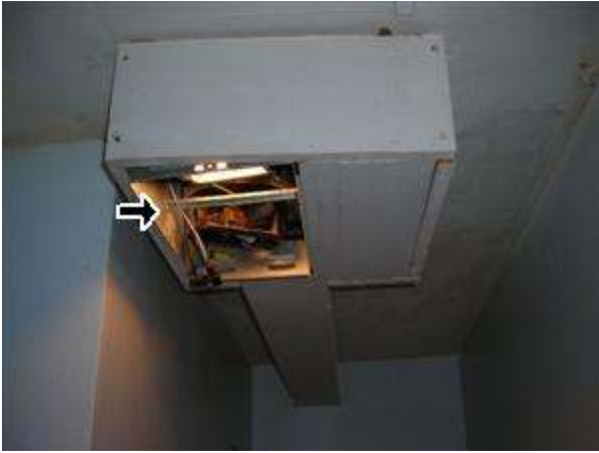
5.8.A Picture 1 Missing cover for bathroom vent.
