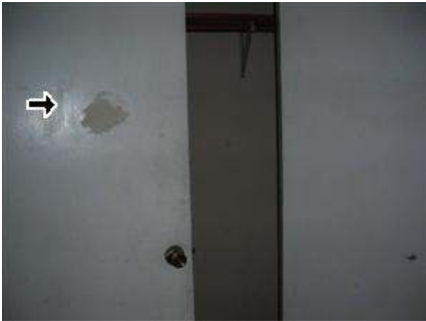
5.3.B Picture 1 Previous repairs to door
