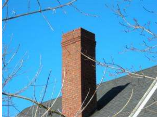
1.2 Picture 2 Some repointing may be required, rear chimney
