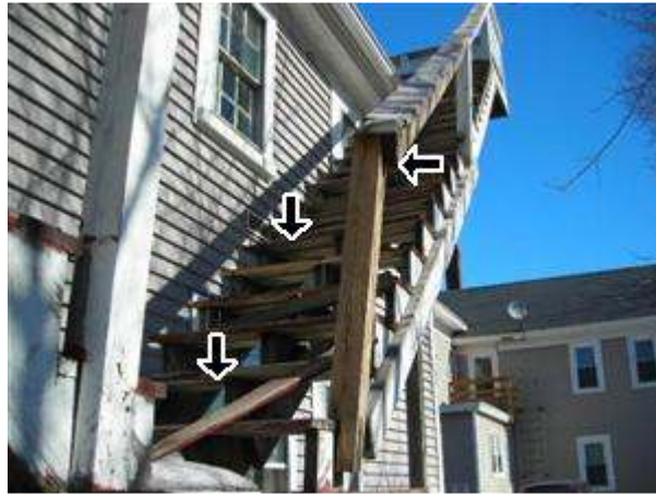
2.4 Picture 4 Staircase is unsafe
