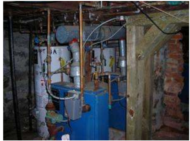
5.17.A Picture 2 Heating and hot water units for 17A & B
