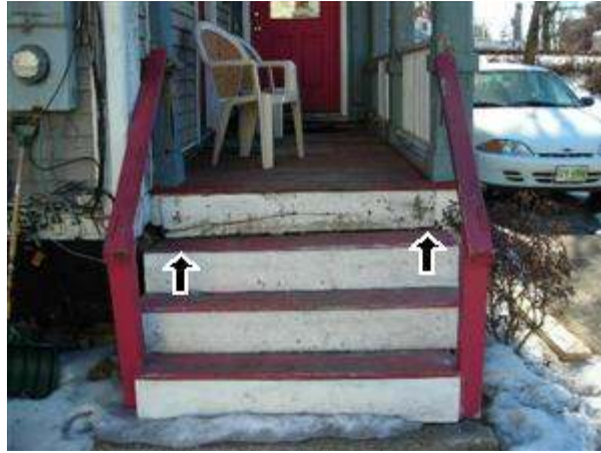
2.4 Picture 8 Steps need repair
