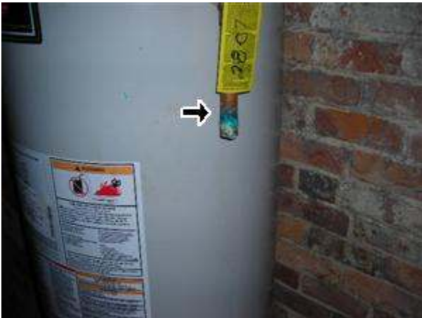
4.2 Picture 1 All water heaters should have the pressure relief valve extend to the floor for safety
