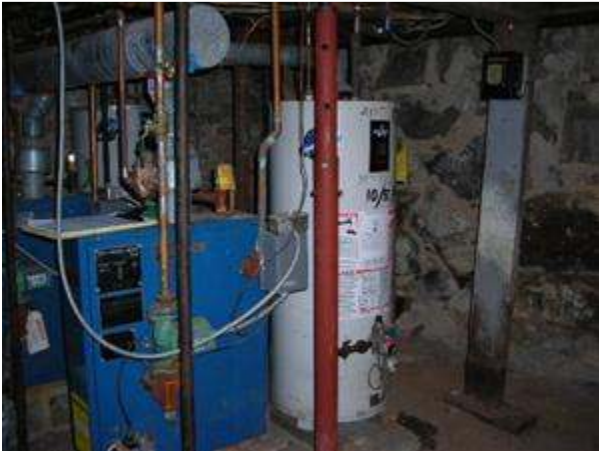
5.17.C Picture 1 Heat and hot water units
