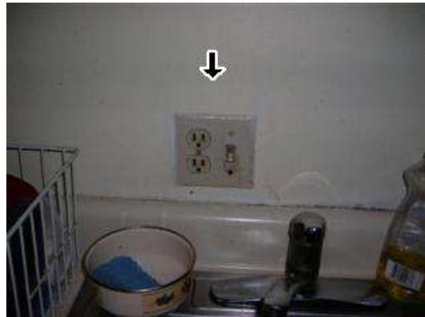
5.9.C Picture 2 No GFCI at kitchen sink
