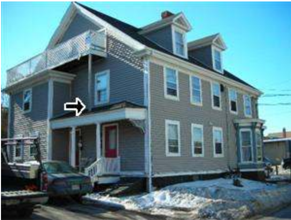
2.4 Picture 1 Deck not supported properly
