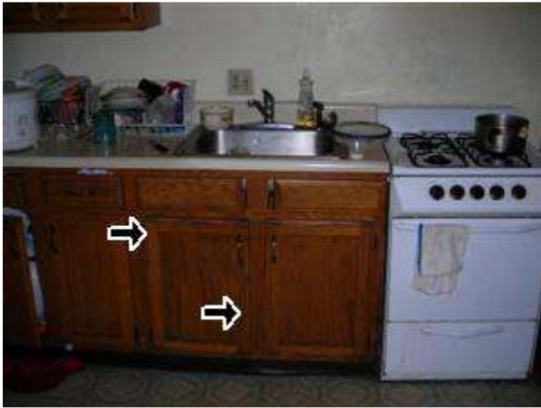
5.5.C Picture 1 Base cabinet and countertop need repair
