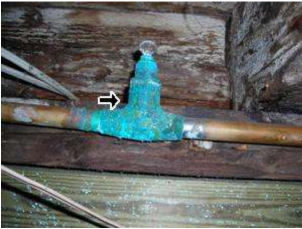
4.1 Picture 1 corrosion on valve near unit 19 heating system, may need repair.
