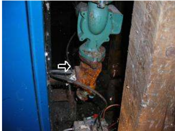
5.17.C Picture 2 Evidence of past leaking
