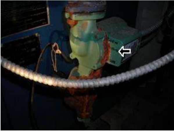
5.17.B Picture 1 Corrosion at the circulating pump
