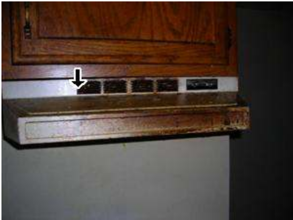
5.8.C Picture 1 Vent for stove
