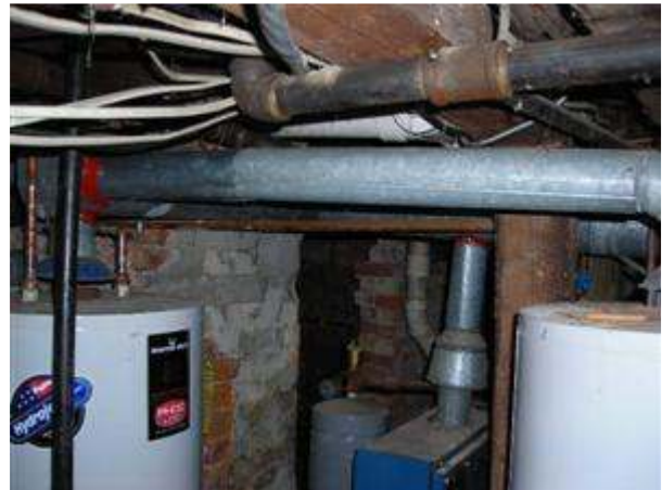
4.2 Picture 2 Water heaters and boiler venting
